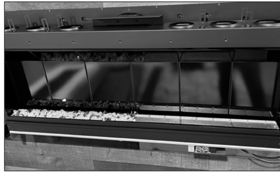
Burner Glass Media partially installed
