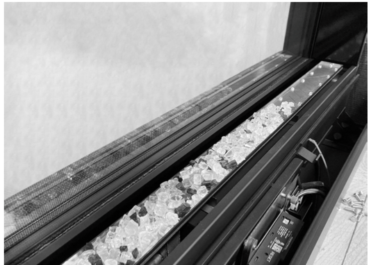
Burner Glass Media – Partially Installed
