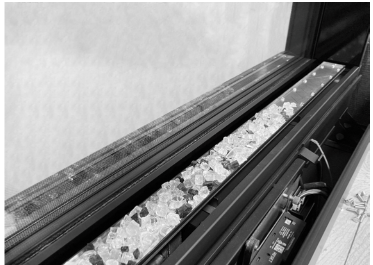
Burner Glass Media – Partially Installed
